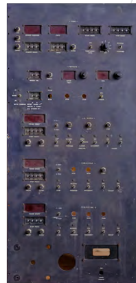
Control Panel Detail
